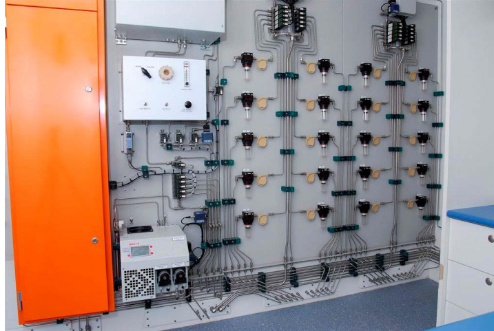
Figure 2.11: Filters and gas measurement unit of tube bundle system [53]
